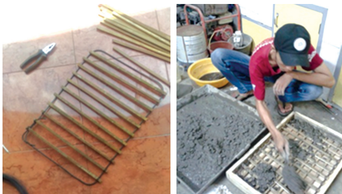
Figure 3: The process of making water gates from panels with reinforcement from bamboo
