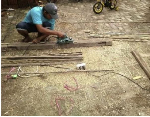
Fig. 6. Exfoliating the inside of the bamboo and adjusting the dimensions of the bamboo to the reinforcement plan.
