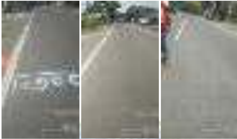
Gambar I.36. Retak Pinggir (Low), Retak Memanjang (Medium), Retak Blok (Low)
