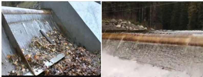
Figure 1 Screen condition of tyrol weir which is sediment
